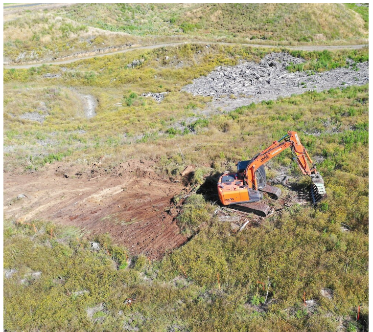
Mechanical clearance using a 14 tonne excavator and rake to enable easier site access and planting.
